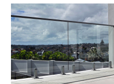
frameless glass balustrade front balconies
